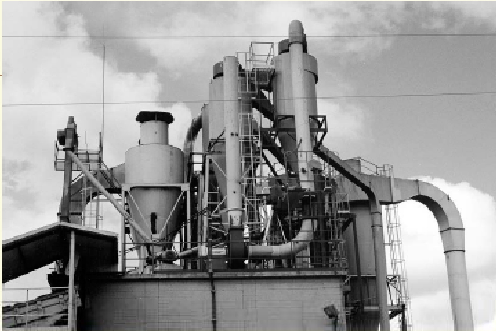
Dust collection cyclone installed in series with the hammer mill cyclone
